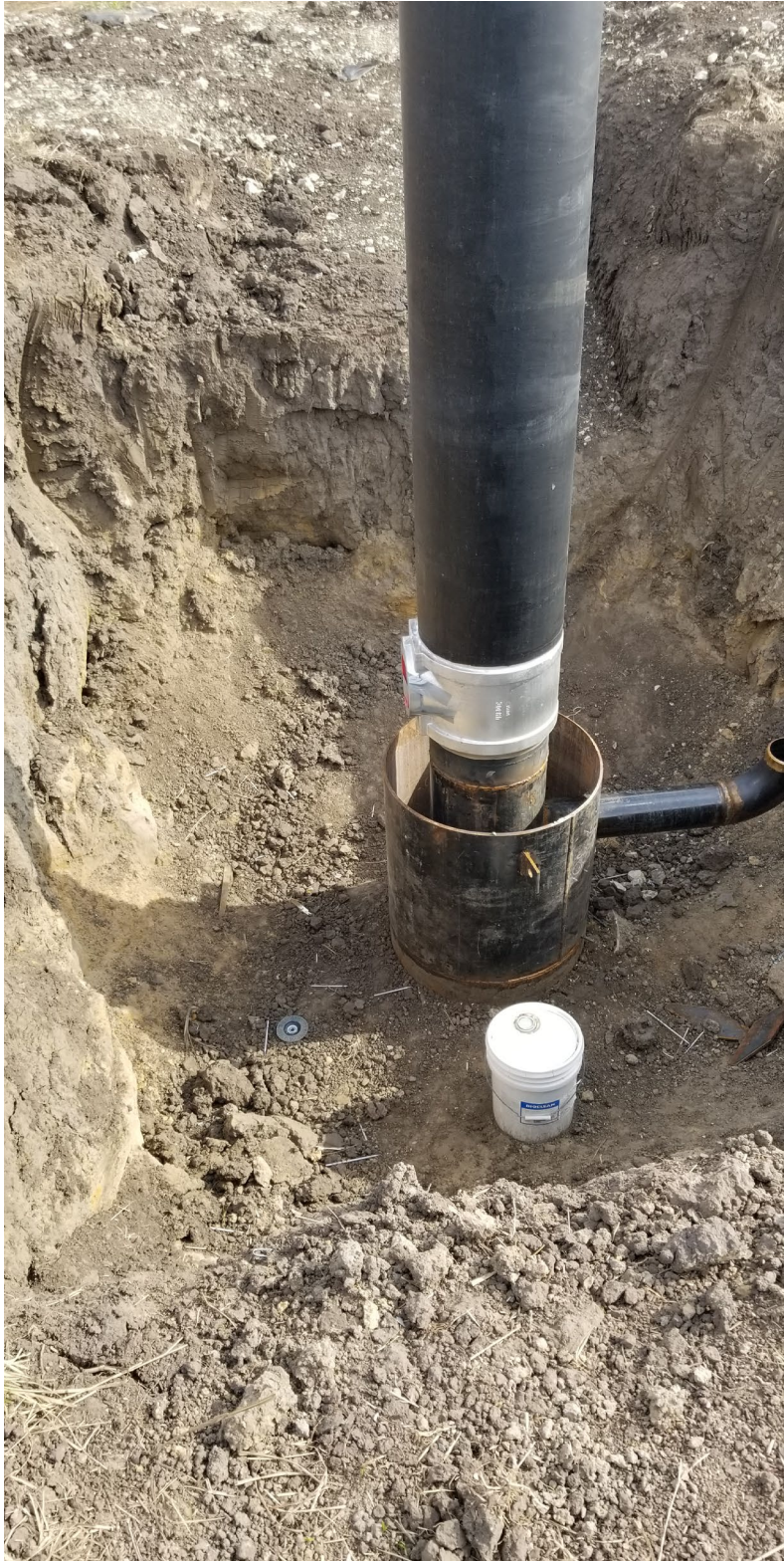
Well #11 wellhead in lower casing.
