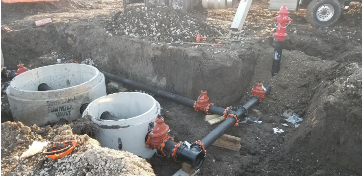
The piping for well #11 has been installed. Excavating the raw water main is in the works.
