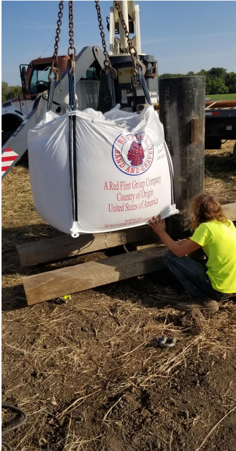
Once the screen was level and centered Brotke staff began installing the well media.
