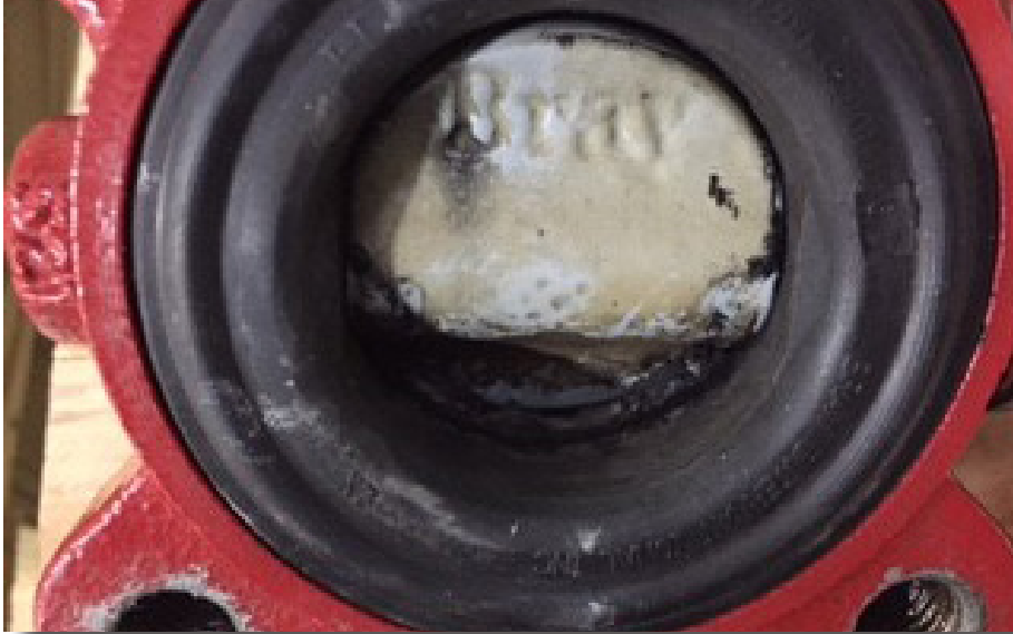
October 12, 2015 – changed valves 105 and 107 to address CIP water level issues.
